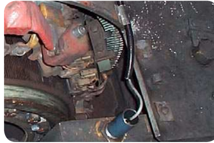
Vibration sensor installation in a Swedish MTAB Dm3 locomotive traction motor/gearbox
