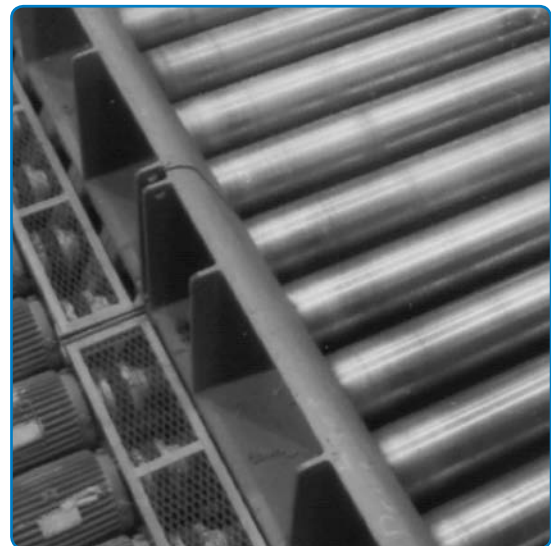
ELASTOMERIC™ Coupling for Runout table (shown under the guard) at a major hot strip steel mill
