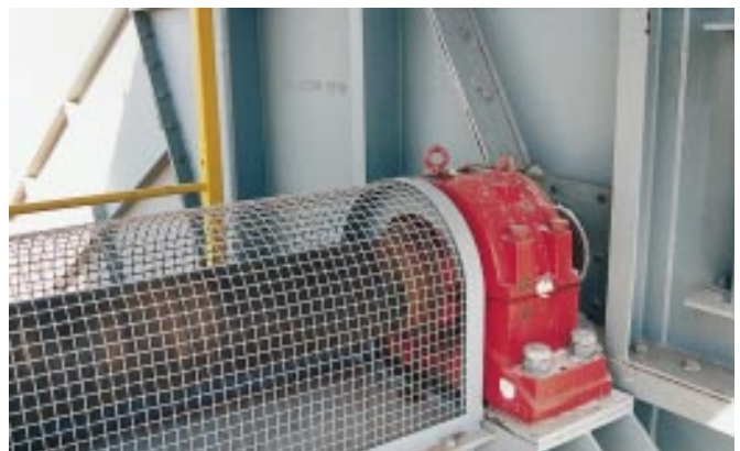
Ventilator drive unit
