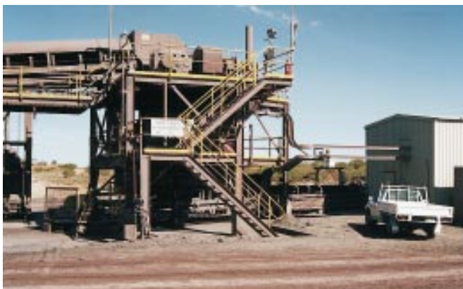
Conveyor plant drive unit
