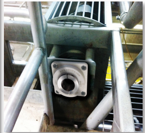
No rust! No grease!
